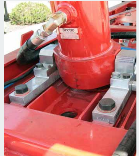
Loadcells mounted under hoist
